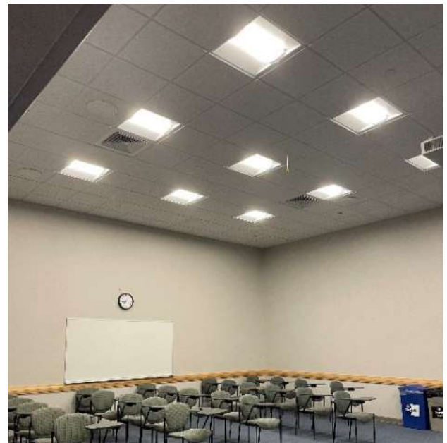
J. Ray Ryan Lecture Hall Room 204 LED Upgrade
